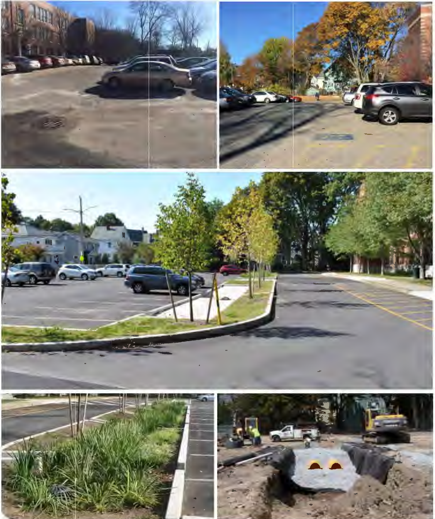
Figure 7. Before and after photos of bioswale and underground chambers in the rear parking lot.
