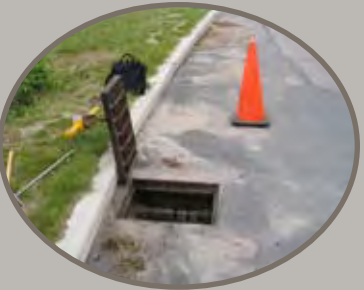
Leaching Catch Basins
