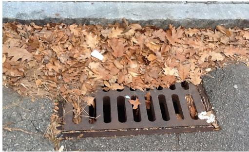
Keeping catch basins clear of leaves and debris lets water flow through Boston's storm drain system.
