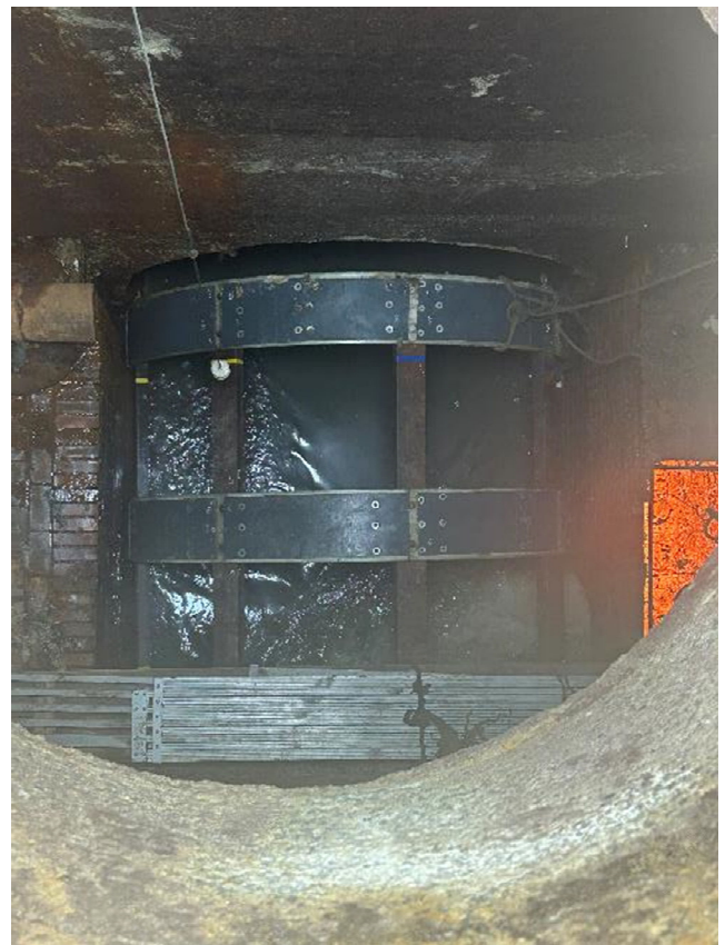
Mandrel is pulled through the NBMI pipe to confirm slipline pipe sizing.
