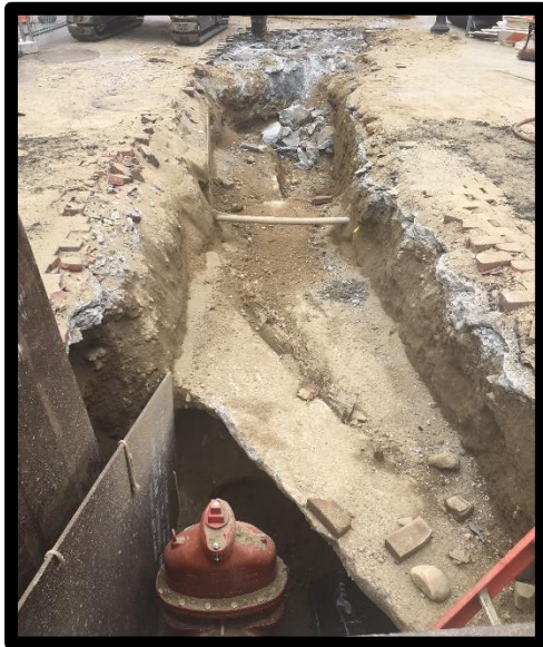
Utility Conflicts During Water Main Installation Cross Street
