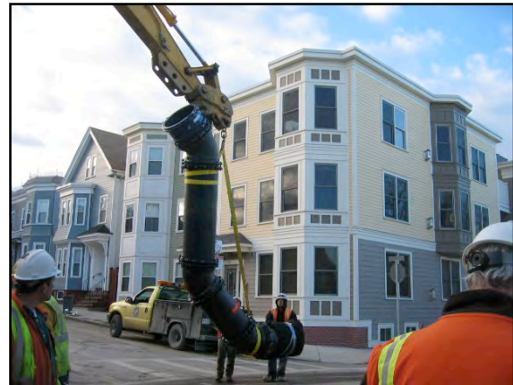
Relocation of 20" water main in East Third Street to accommodate installation of 36" drain.
