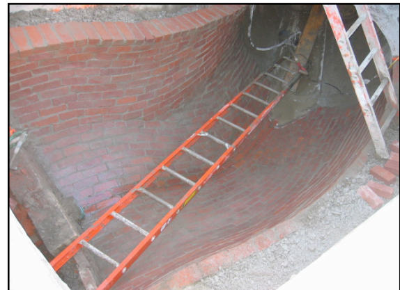
New brick invert in MH D between the new 66" storm drain and existing tidegate in Farragut Rd.
