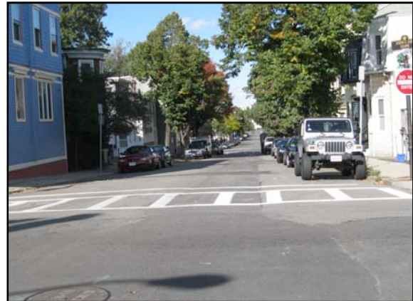
Completed intersection of East Second Street and O Street showing temporary paving, in anticipation of permanent paving.
