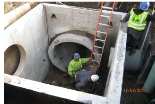
Installation of Special Manhole C at West First Street and F Street
