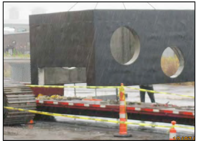
Special Drain Manhole C being delivered for installation at the intersection of West First Street and F Street
