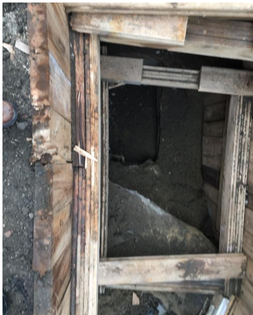
Phase II Utility Conflict
