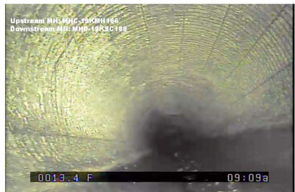
Extensive corrosion in 36" pipe in Dorchester Avenue to the NBMI, which is being rehabilitated.
