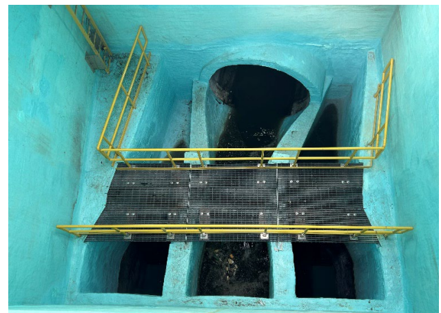
Special Manhole E, rehabilitated with cementitious liner and epoxy coating and ready for safe access.
