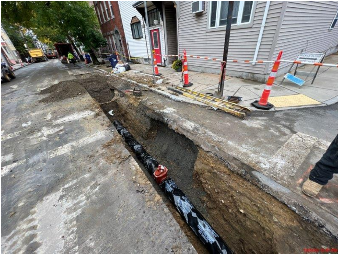
Cottage St – 8-inch ductile iron, zinc coated class 56 pipe with 8-inch gate valve. Poly wrapped with V-Bio Polyethylene Encasement to inhibit corrosion.
