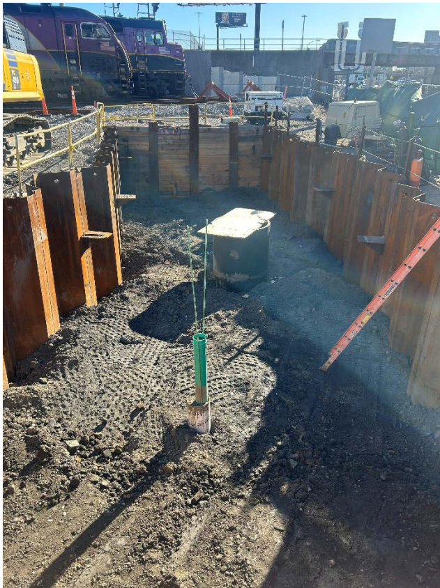
Jacking pit is backfilled in lifts and manhole riser is installed as backfilling progresses.
