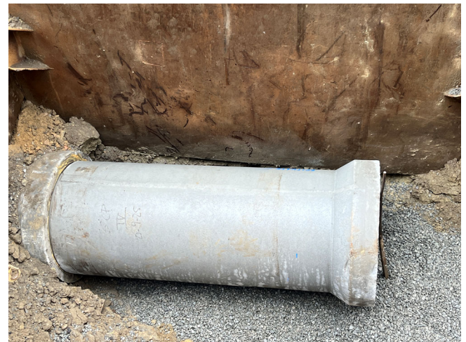
Drainpipe in West Fifth Street
