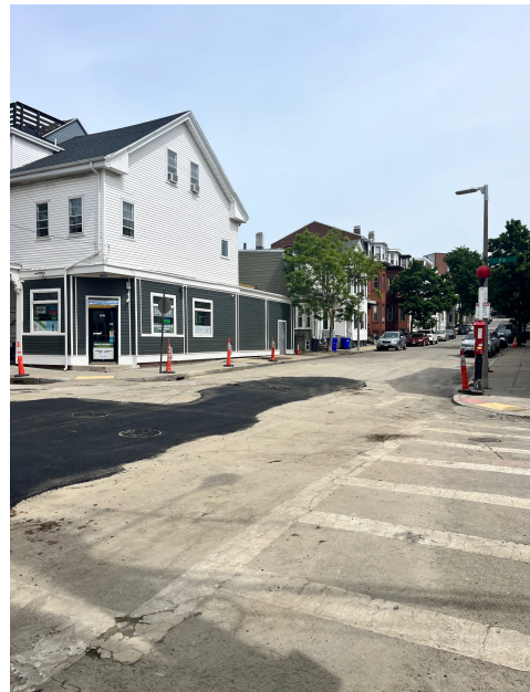
Temporary paving at the intersection of West Fifth Street and F Street
